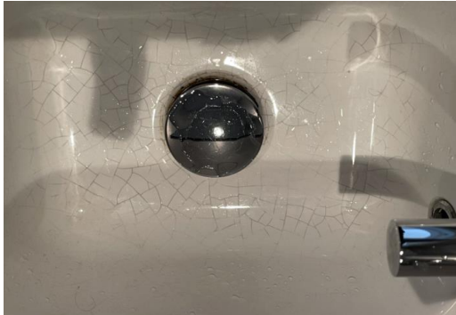
Krakelering i servant
